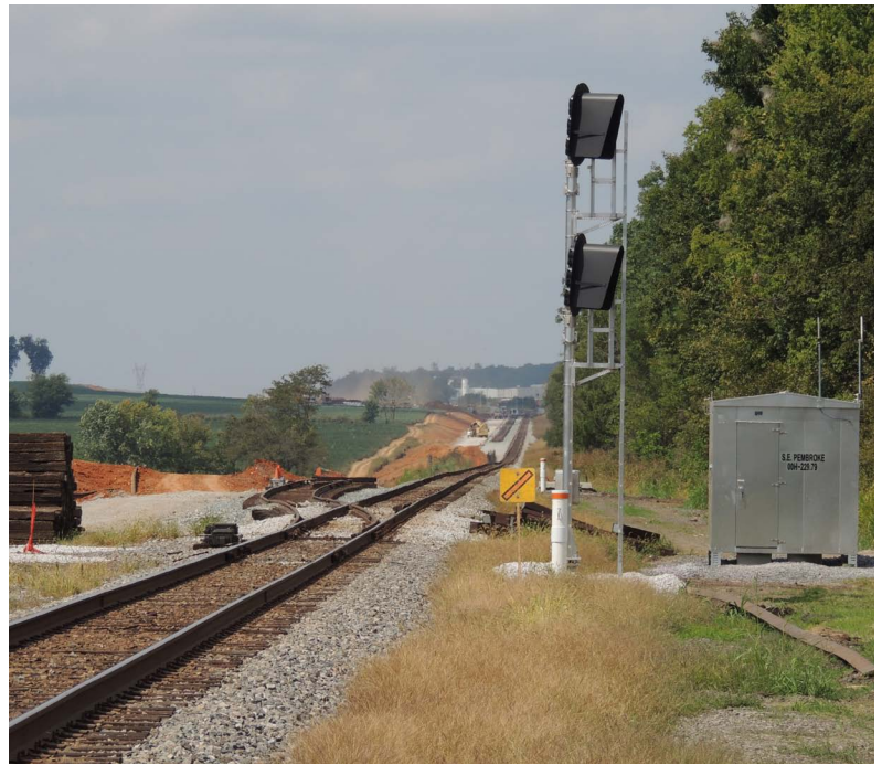
Above: The new signal and switch at South Pembroke. This is the South end of the Casky yard lead. - Thomas Bryan
